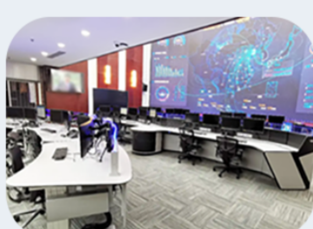
CONTROL AND COMMAND CENTER
